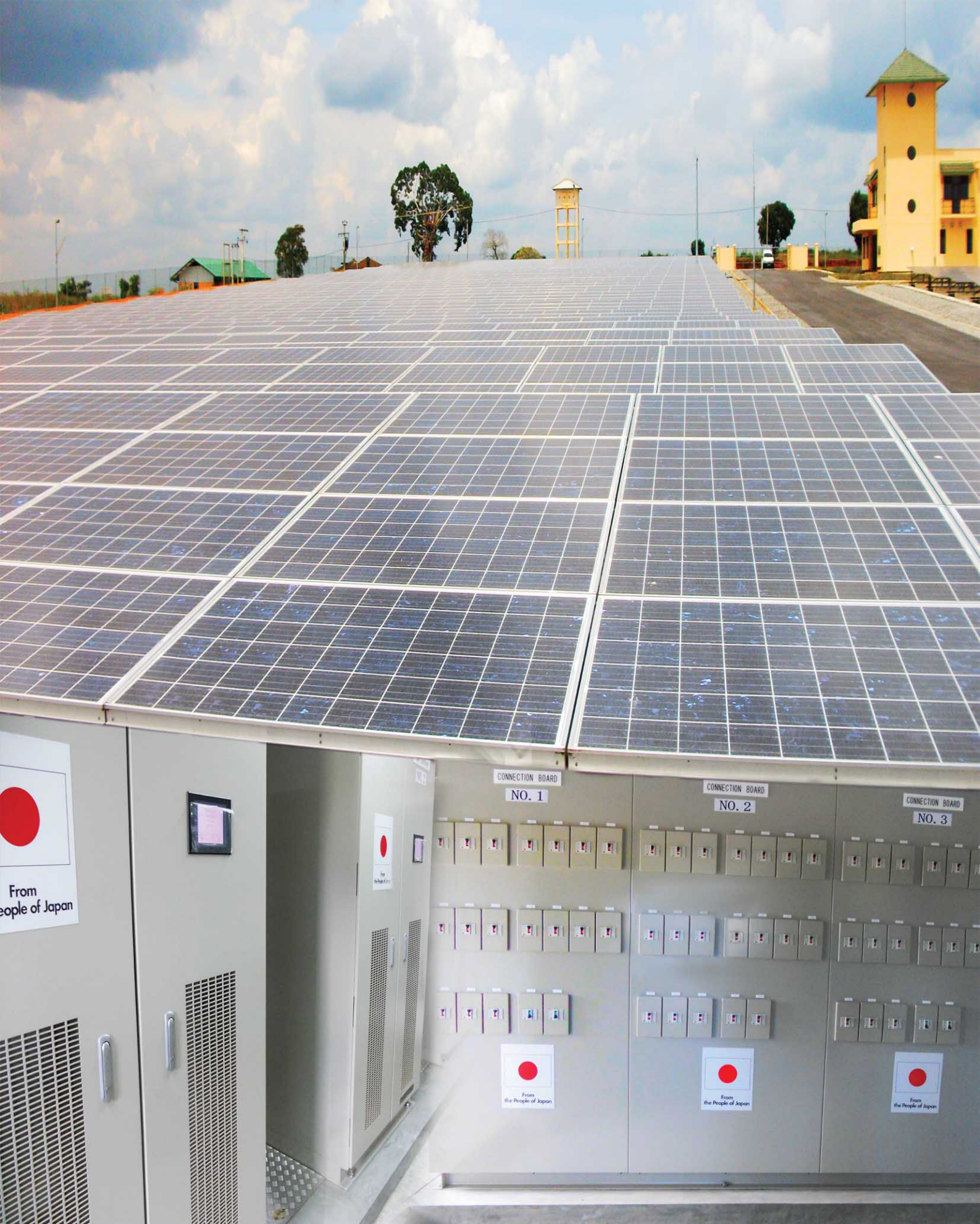
Electrical and Mechanical Contractor for Sri Lanka's Largest Solar Power Generation Project.
